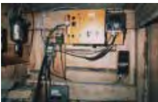
Gas drainage monitoring sensors
